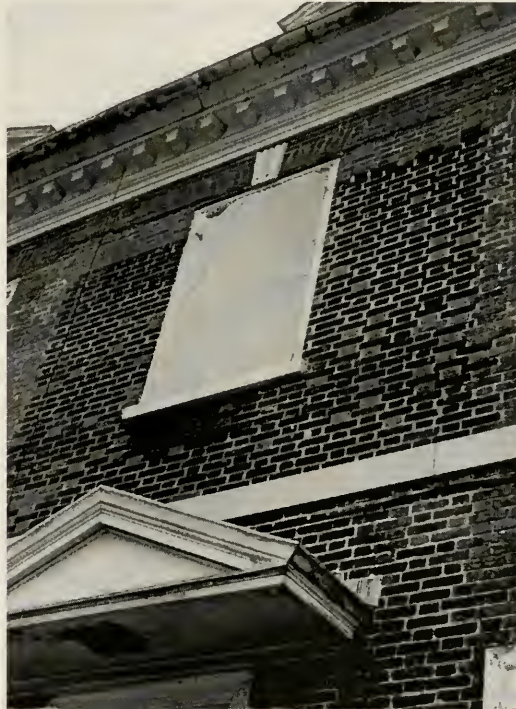
Figure 26 Inappropriate Masonry Infill, 1998 Photograph by Author
